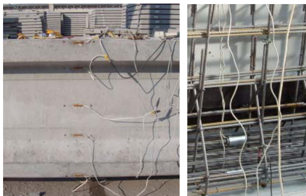
Fig. 4b) Strain gauges and elastomagnetic sensors
